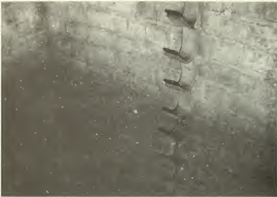
Photograph no. 62: Interior of Feature 7 showing hangars for high voltage electrical wiring
