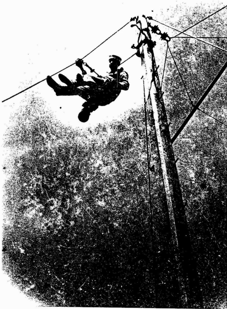
C. W. Mulligan, in boatswain's chair, applying red lead to guy wires. Salt accumulation cleaned periodically from insulators to prevent arcing. Point Montara, NLH, 1921.
