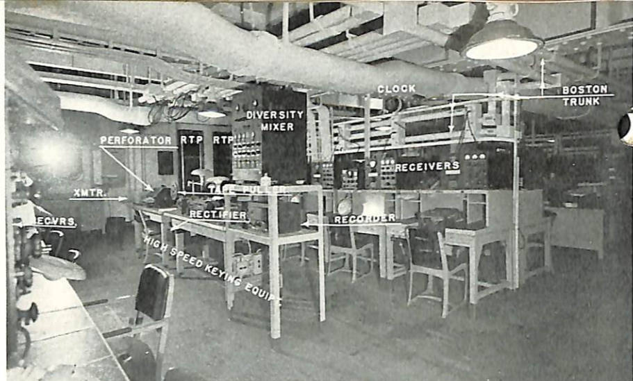
Port side of Radio I, showing high-speed c-w communication and miscellaneous equipment.
