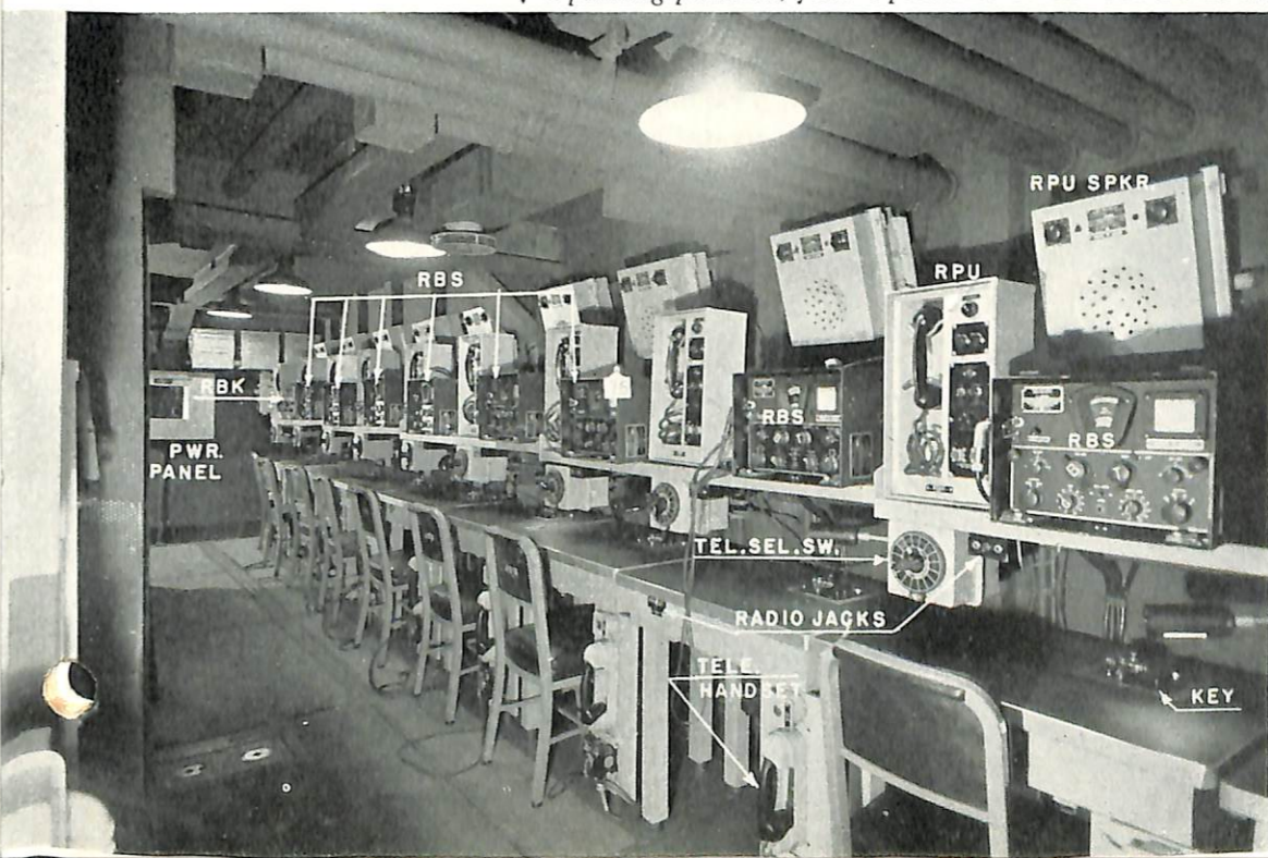
▼ Operating positions, Joint Operations Communication Room.
