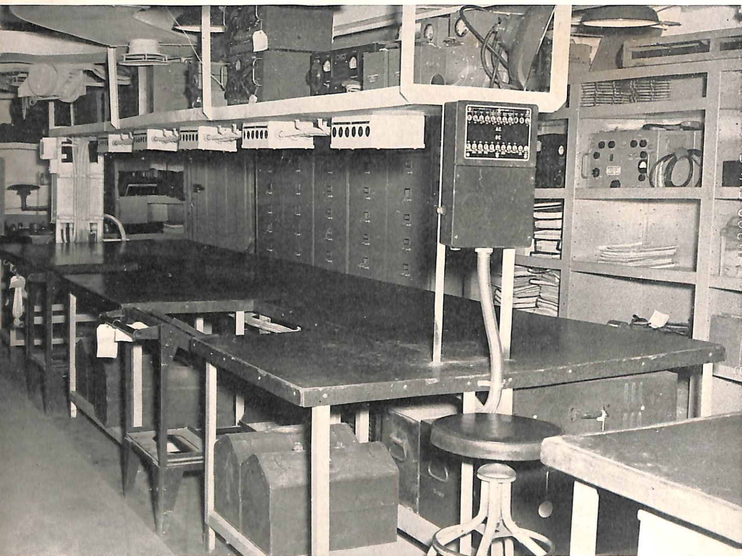
The AEW radar workshop. Note the numerous facilities, convenience outlets, large work benches, test equipment, etc.
