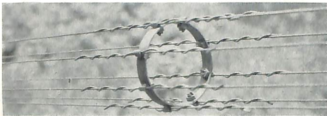
DOWNLEAD CONSTRUCTION, the new method, showing preformed springs used to prevent move of downlead wires at point of attachment and resulting crystallization.
