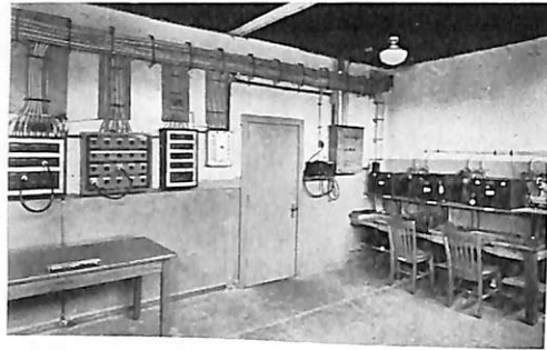
RADIO OPERATIONS, showing transfer panels and cabling (USNR Training Center, Clifton, N. J.)
