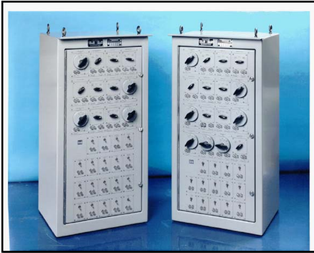
Figure 3-27.—Local IC Switchboards.
