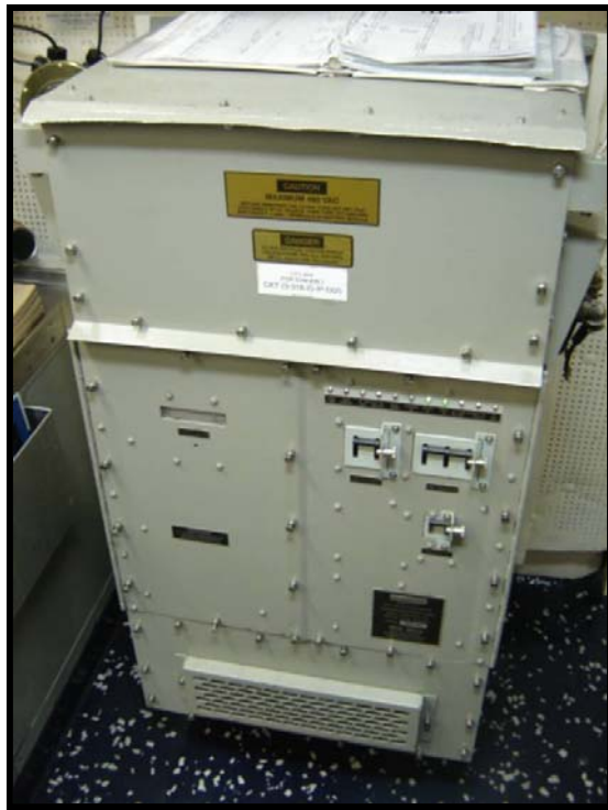
Figure 7-27.— 2kVA 1MC UPS.
