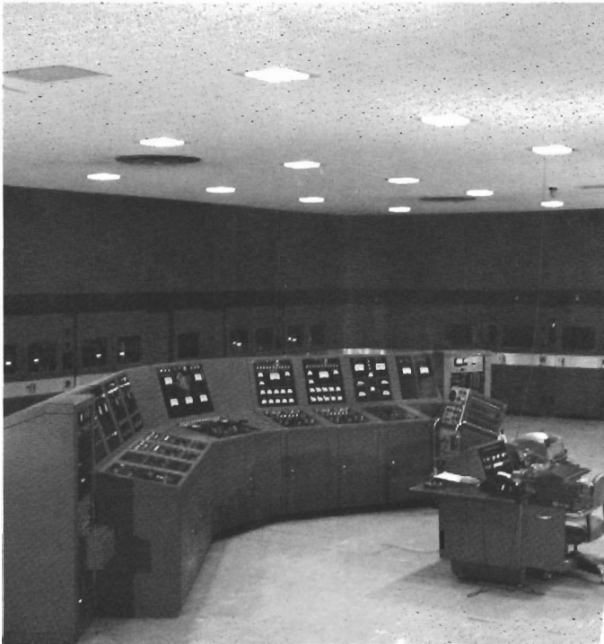
VLF CONTROL CONSOLES AND TRANSMITTER, NAVAL COMMUNICATIONS STATION, CUTLER, MAINE
